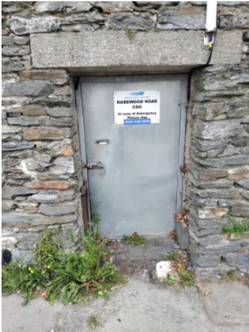
South West Water’s Combined Storm Overflow on Harewood Road
